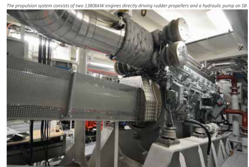
The propulsion system consists of two 1380kW engines directly driving rudder propellers and a hydraulic pump on SB
