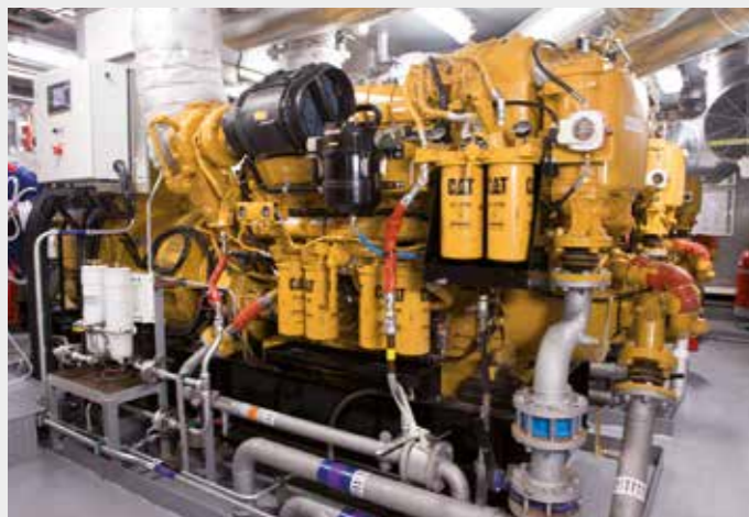
The diesel generator sets are freshwater-cooled Caterpillar units
