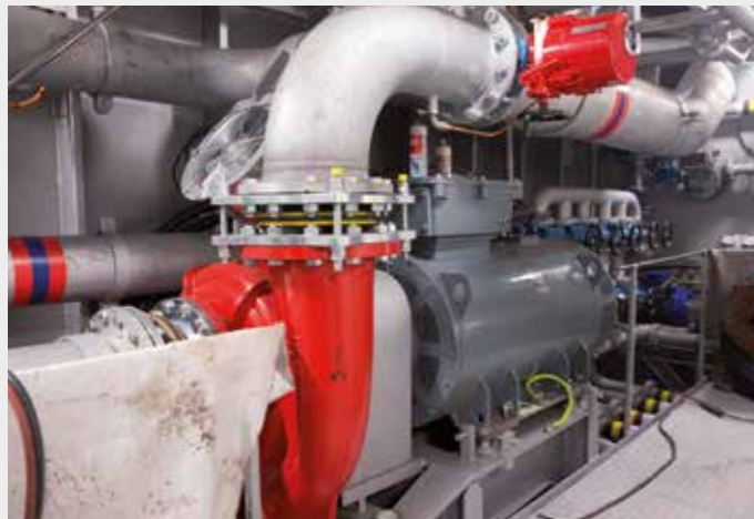
The waterspray system is fed by the dedicated Fi-Fi pumps in the aft ship
