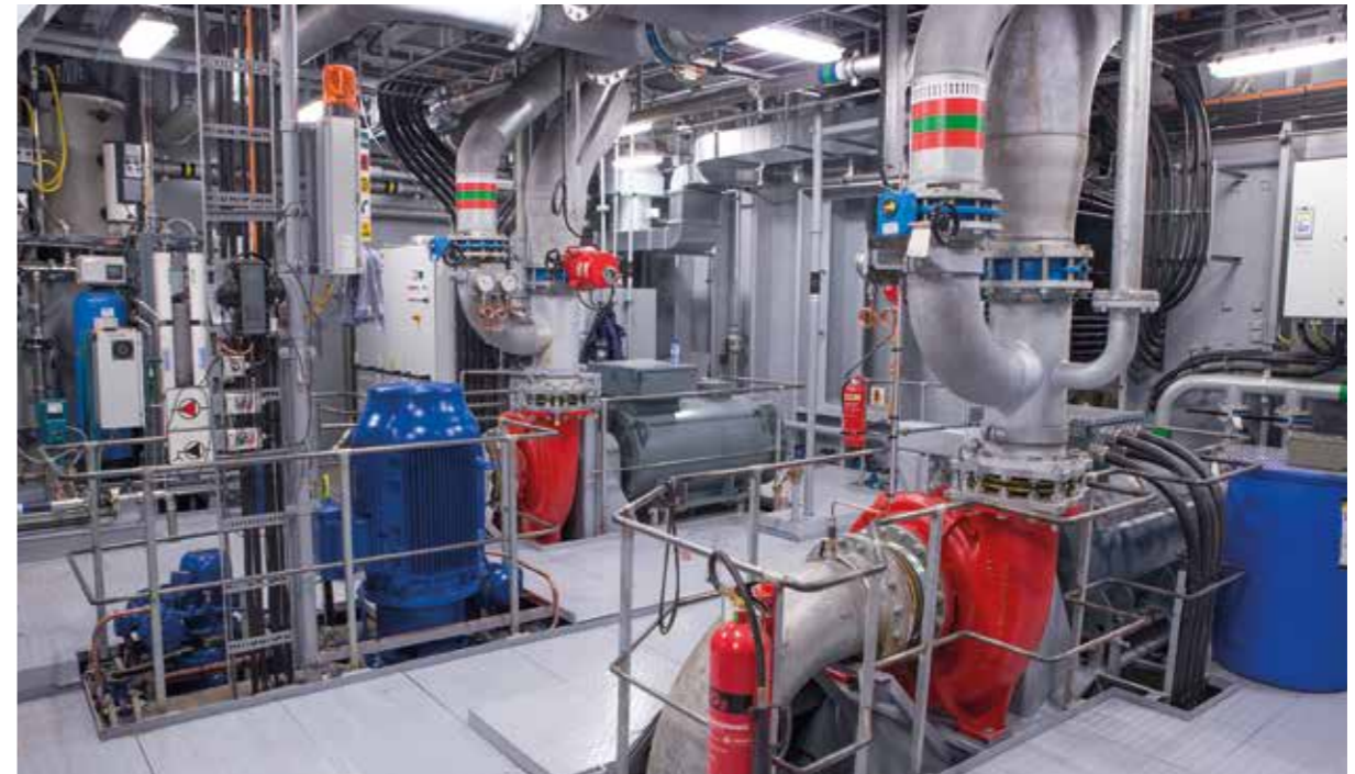
For external fire-fighting purposes, monitors are fed with water from two dedicated electrically driven Fi-Fi pumps
