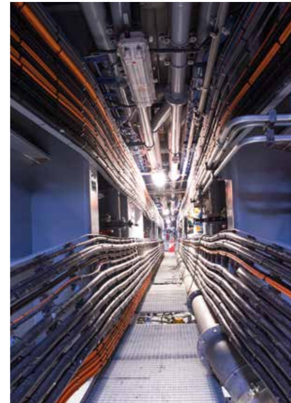
Power cables and piping running through the longitudinal corridor between the pump rooms
