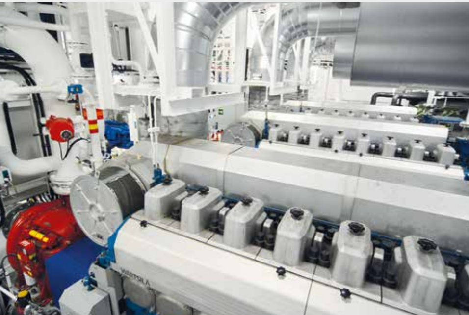
The three main generator sets of 1480 kW each, are driven by medium speed engines
