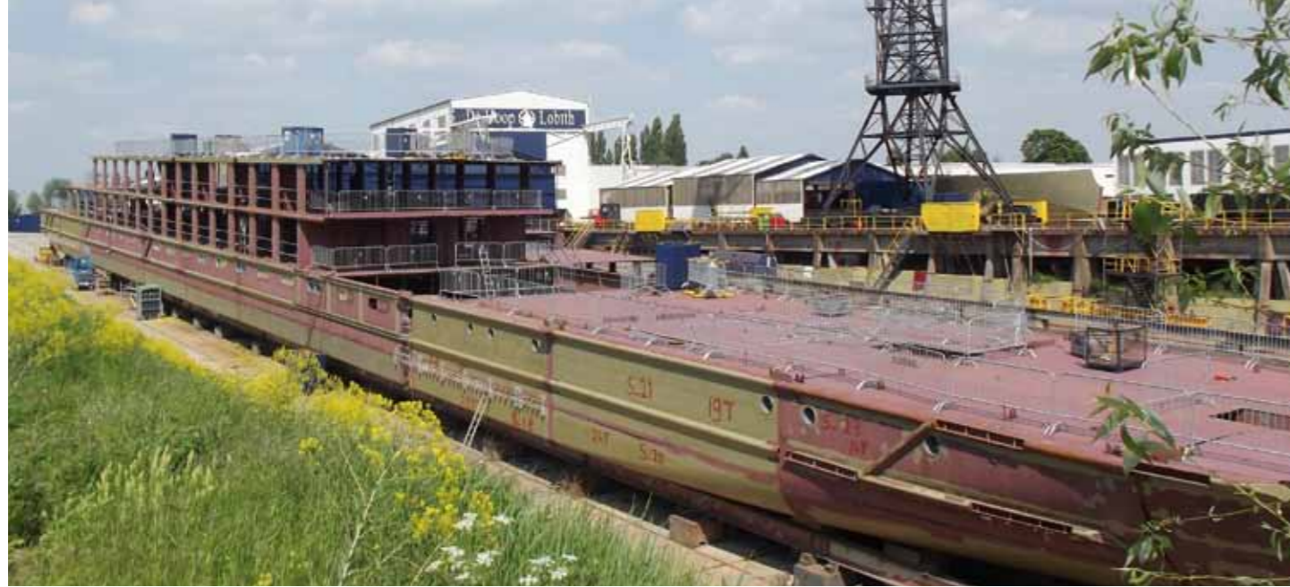
De Hoop slipway facilities, for vessels up to 200 metres length, offering all disciplines to build a complete ship
