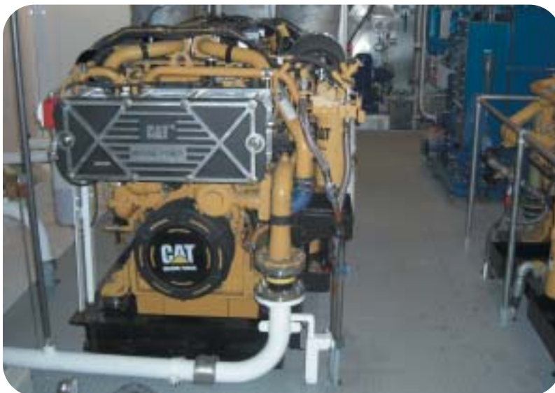
Pon Power supplied the main and auxiliary engines and generator sets
