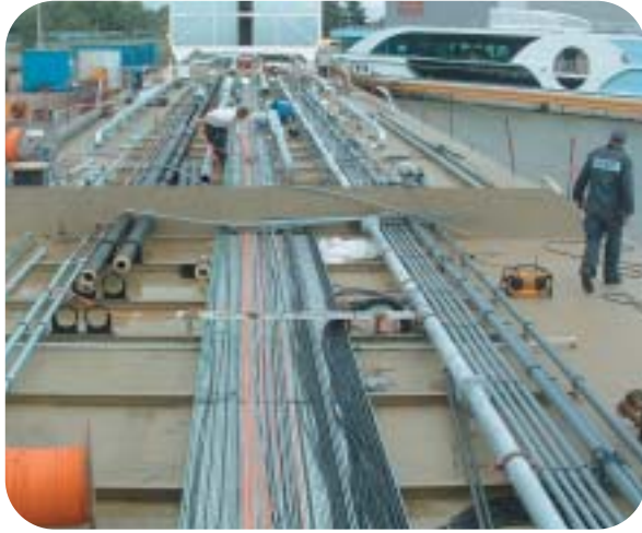
The 1.2 m high technical space above the main deck proved essential in achieving the speedy delivery
