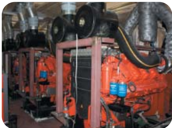
Three Veth gensets provide onboard power
